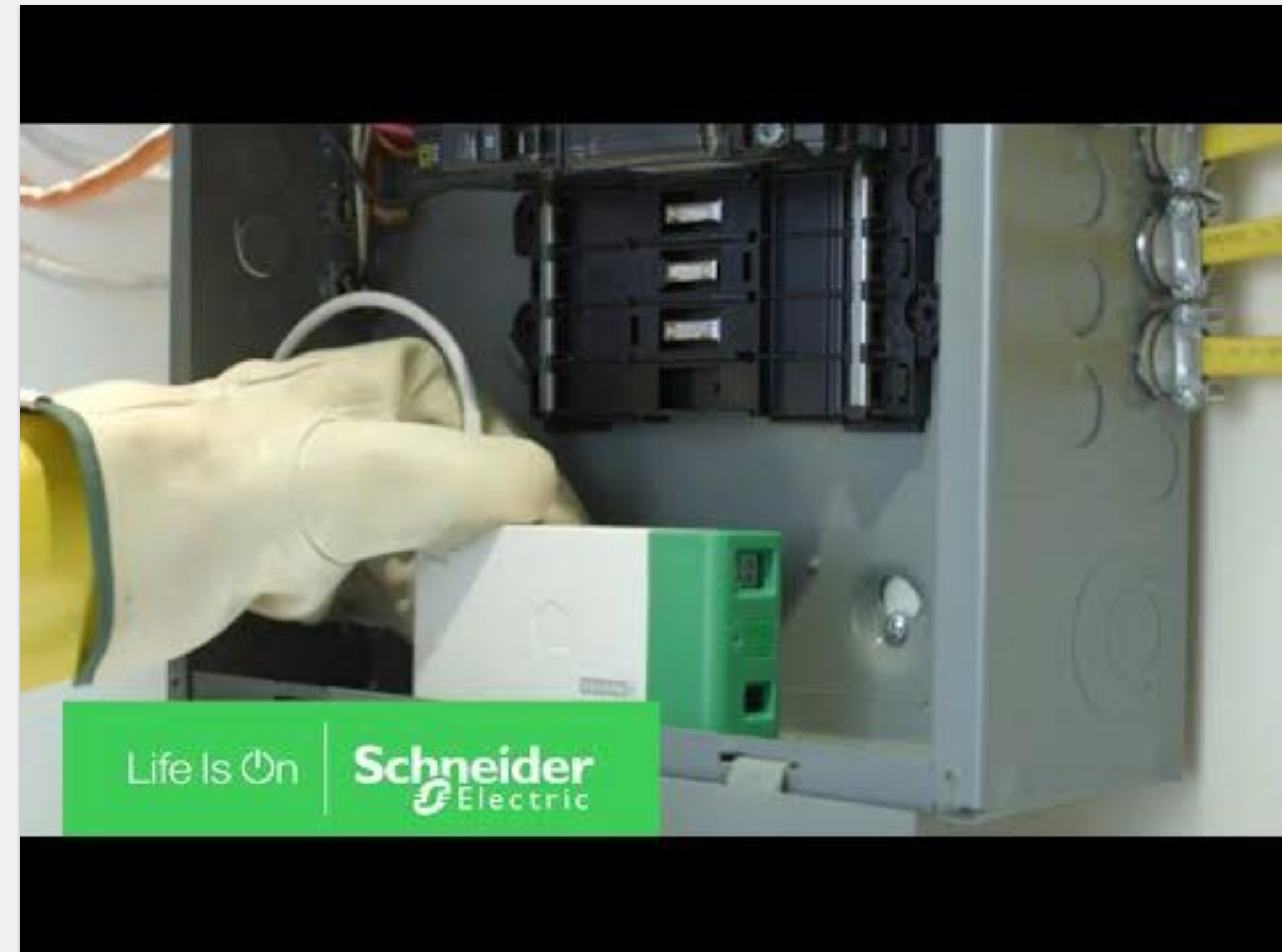
Demonstration of how to install the device and allow it to monitor energy usage
